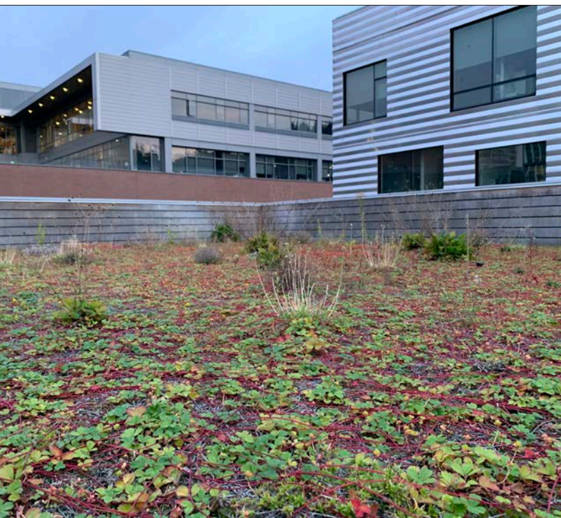
Figure 37—Green roof at Portland State University. (Photograph by Matthew Shepherd.)
