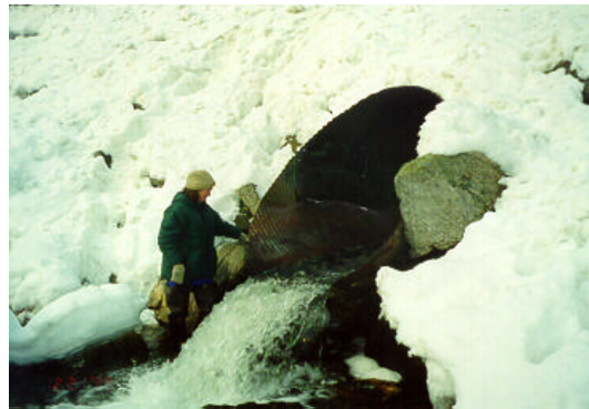
Figure 1. Example of a culvert that may not allow upstream passage of some macroinvertebrates. The outflow of this culvert is above the downstream water level because either (1) it was designed and installed this way or (2) downstream erosion has cut the stream's substrate out from underneath the outfall.
