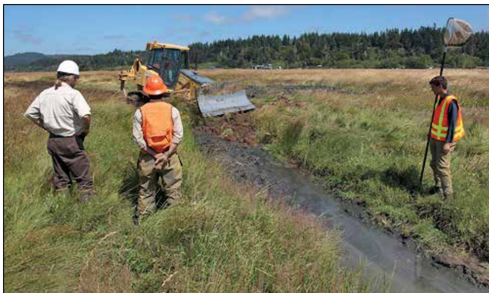
Old drainage ditches were filled slowly to ease fish downstream out of the construction area. USFWS and Oregon Department of Fish and Wildlife biologists monitored the work, capturing and relocating fish when necessary. Photograph by Roy W. Lowe, USFWS.
